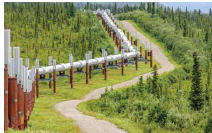
The Alaska Pipeline.
